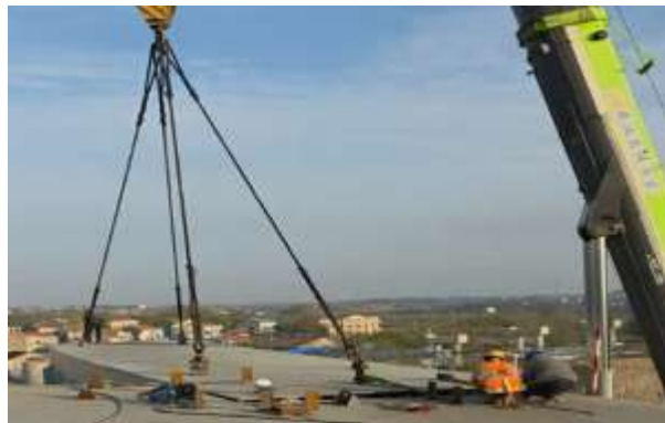
(b) GNSS and other sensors deployed on box girder
